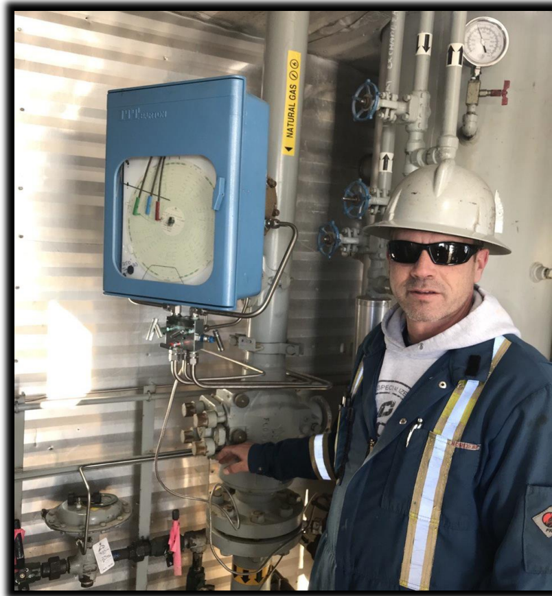
Gas Conservation Operator, Collin Fischer, described and illustrated the pressures, intake, and metering of sales gas from the site project.
