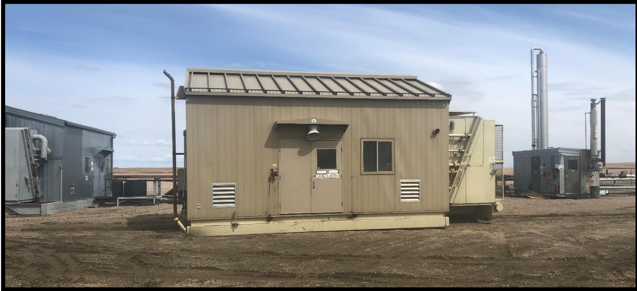
Figure 2 Compressor Station with Dehydrator
