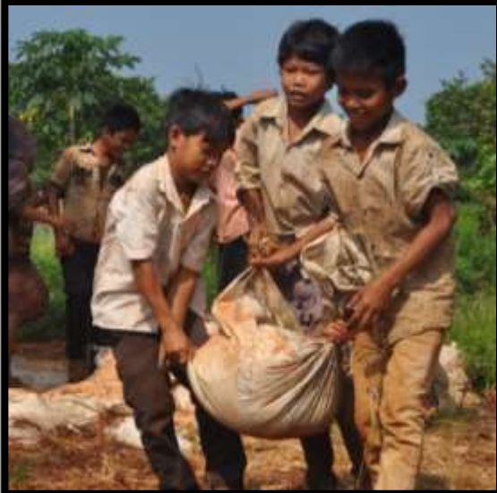
And although not our intention, the students came every day to the site after class and asked to help....
